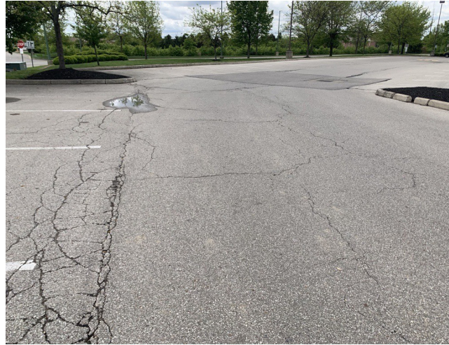
Example of pavement distress
