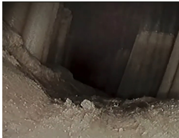
Sediment in tank
